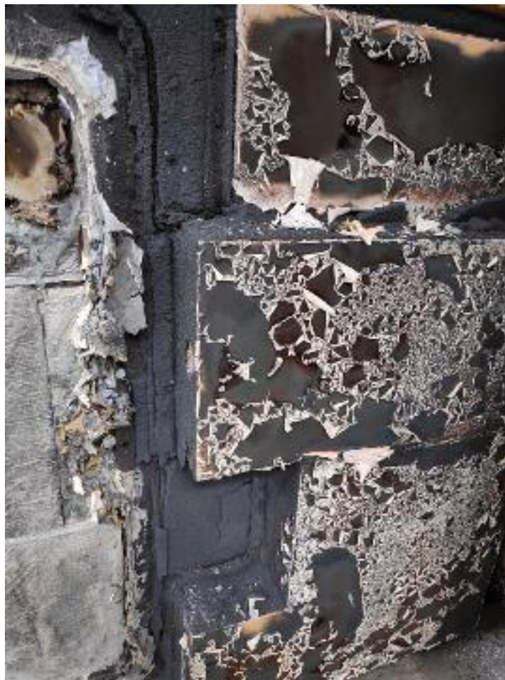
Fig. 8. Burning detail after the test (exposed side).
